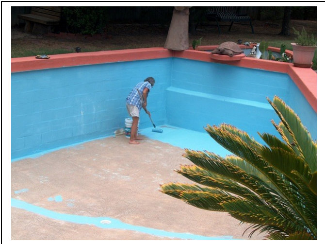
Mother starting on the floor, which was perfectly dry and prepared to receive the paint. Several good coats were needed as the bare concrete really soaked up the first coat.
